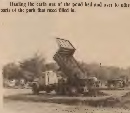
Dumping the dirt so it can later be used to fill in the low spots.
